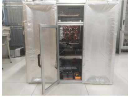
(b) Ventilation door.
