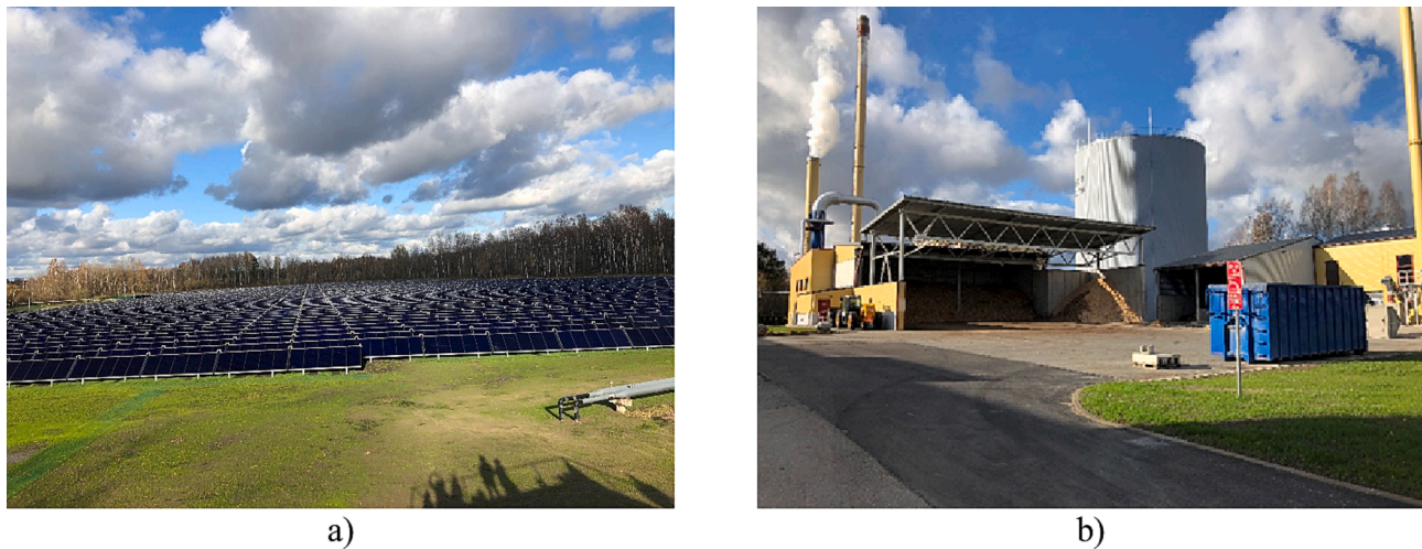
Fig. 1. Solar collectors' system (a) with TES and woodchip boilers (b).
