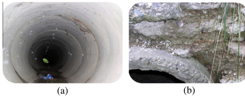
Figure 3 (a) Misalignment of the culvert. (b) Failure of the headwall due to heavy spalling.
